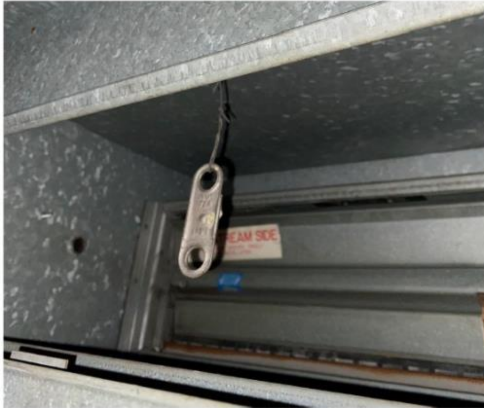
Non-compliant Damper Test
