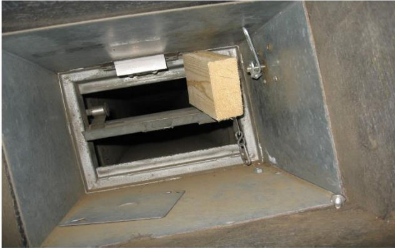
Noncompliance Damper Testing
