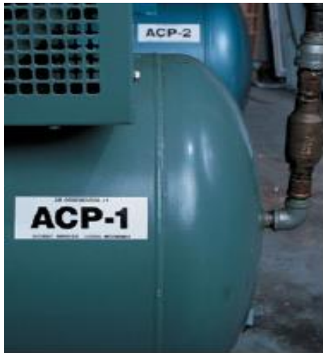
AIR COMPRESSOR #1 ACP-1 DISCONNECT: SWITCH 237
