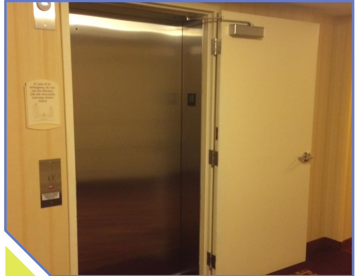
Noncompliant due to not being a tested Assembly
